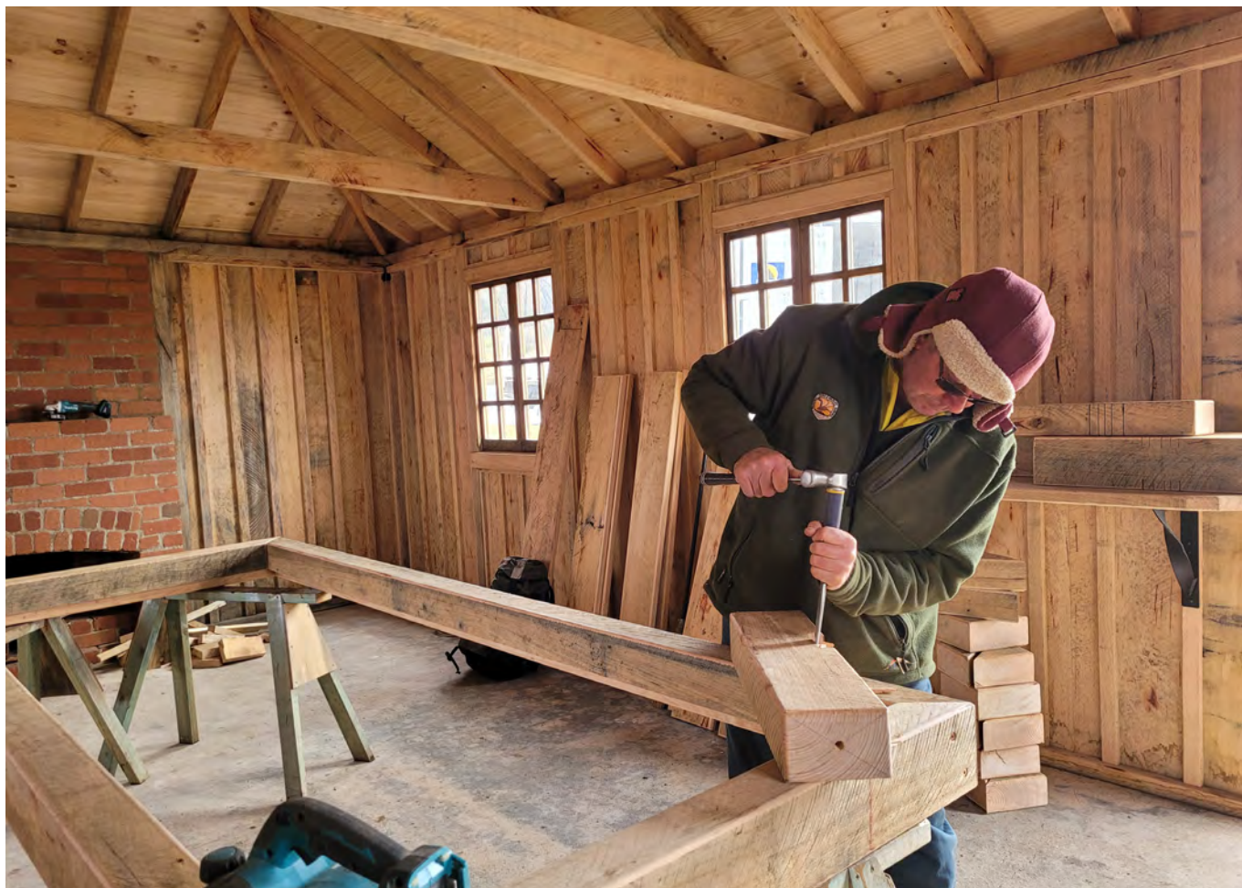
Volunteers and NPWS work together to complete Sawyers Rest Hut. Photo: M Bowden/EES
