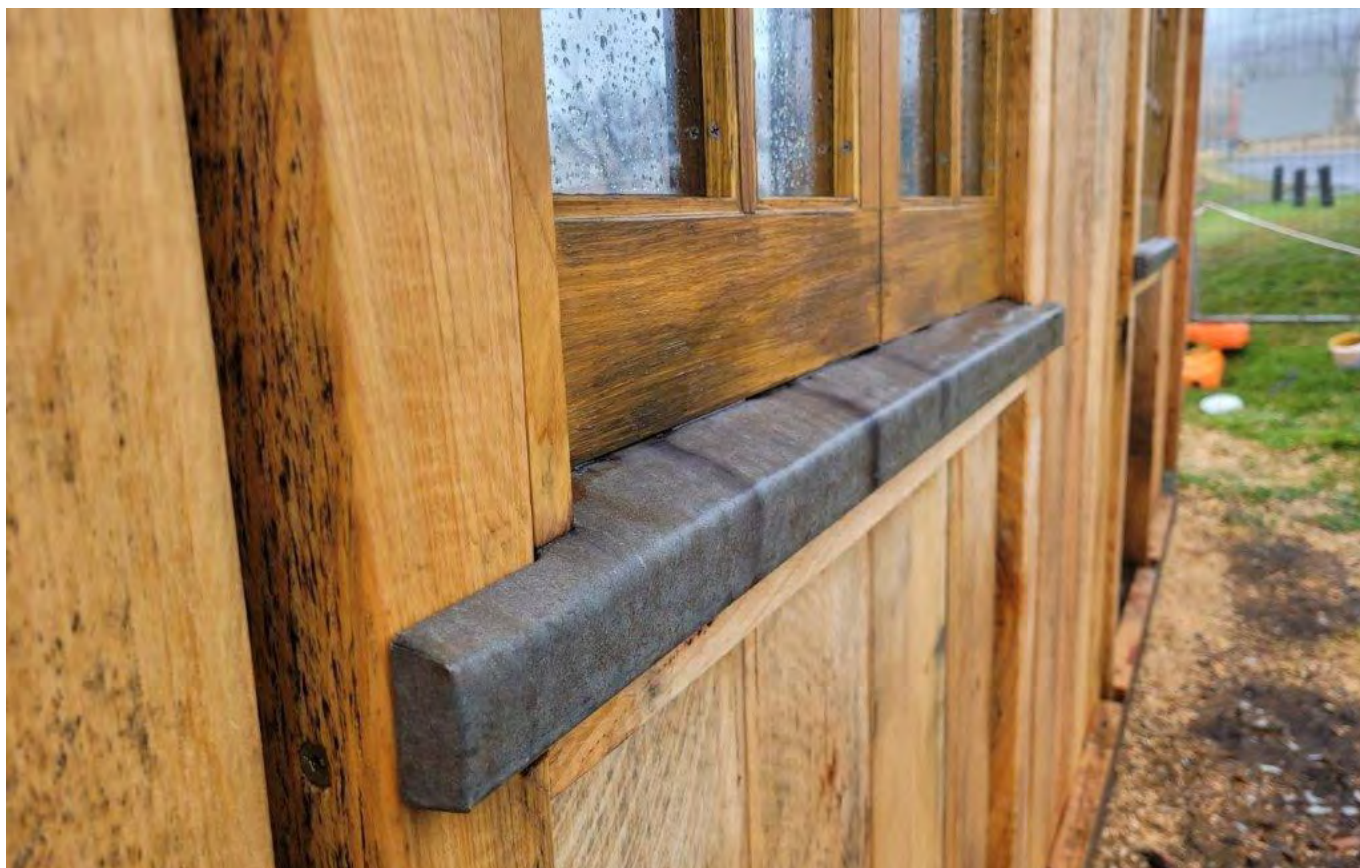
Fire resistant strategies were used including wrapping the windowsills with iron and installing sprinklers. Photo: M Bowden/EES
