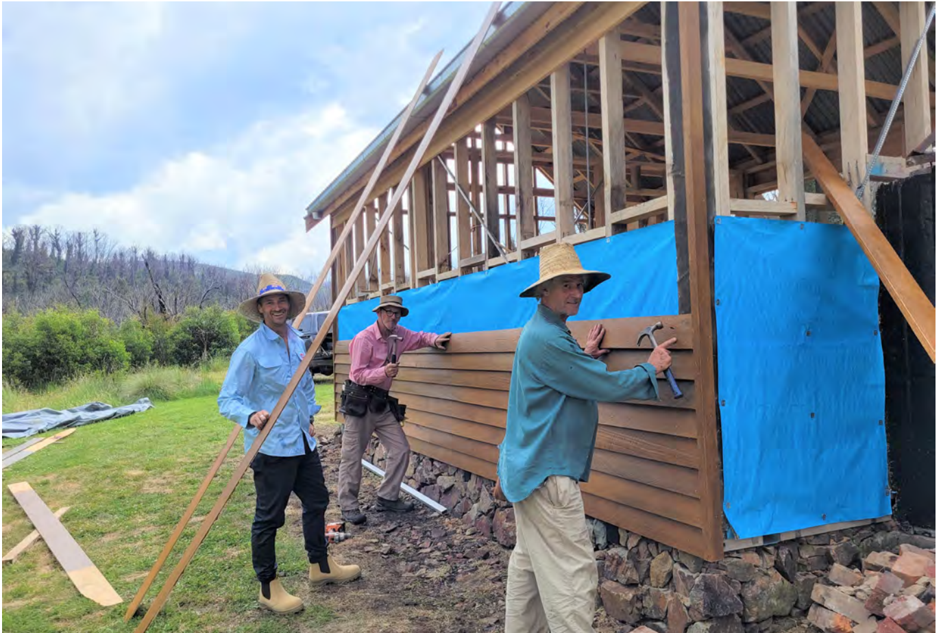
Paul Delany and volunteers installing weatherboards to Delany's Hut. Photo: M Bowden/EES
