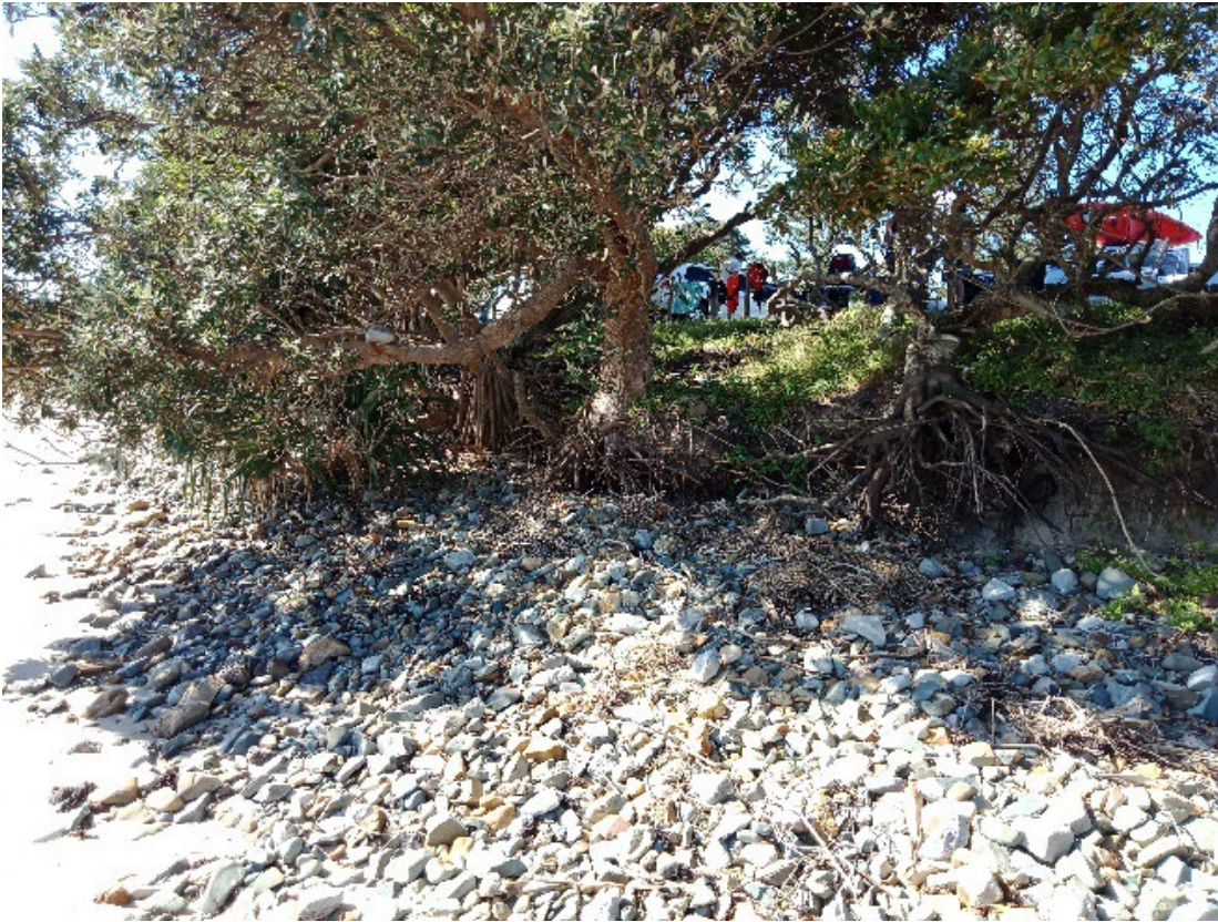
Photo 11 Riverbank erosion occurring approximately 15 metres north of access stairs, Sandon River campground, 2023
