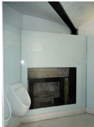
(f) Room B14 looking east, showing raised floor and false walls in front of fireplace
