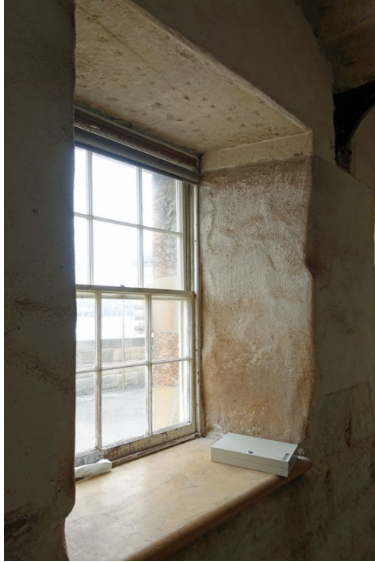
(a) Window in Room B4 showing oil damage to plaster reveals (2018)
