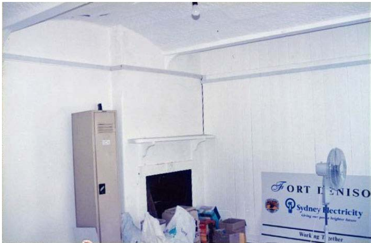
Figure 47 Room B9/B10 before conservation, showing timber partition, picture rail and solid fuel stove in front of later fireplace (NPWS 1997)
