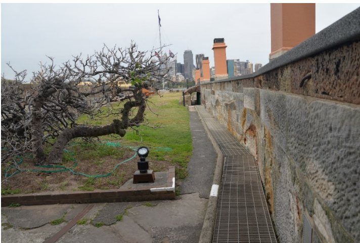
Figure 64 View south-west along the battery, showing the c.1923 drain installed against the barracks to prevent rising damp in the walls. An early 20 th century garden bed (with fig tree) is in the foreground (Casey & Lowe 2018)
