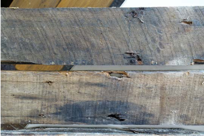
Figure 33 Underside of floorboards from access hatch in Room B6/B7, showing pit-sawn board below and circular sawn board above (Orwell & Peter Phillips 2018)
