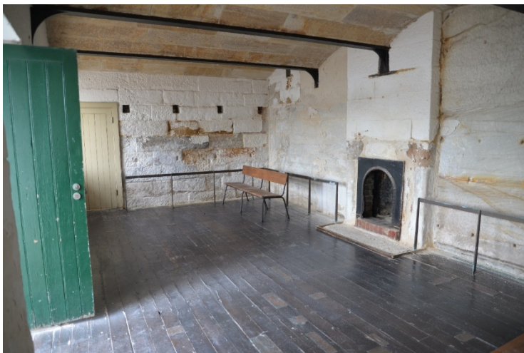
Figure 71 Interior view of barracks Room B5 looking east. Excavations were undertaken in this room during 1997–98 and consisted of the complete removal of floorboards and all subsurface deposits. The room was used as dining space for the café/restaurant until mid-2017 (Casey & Lowe 2018)
