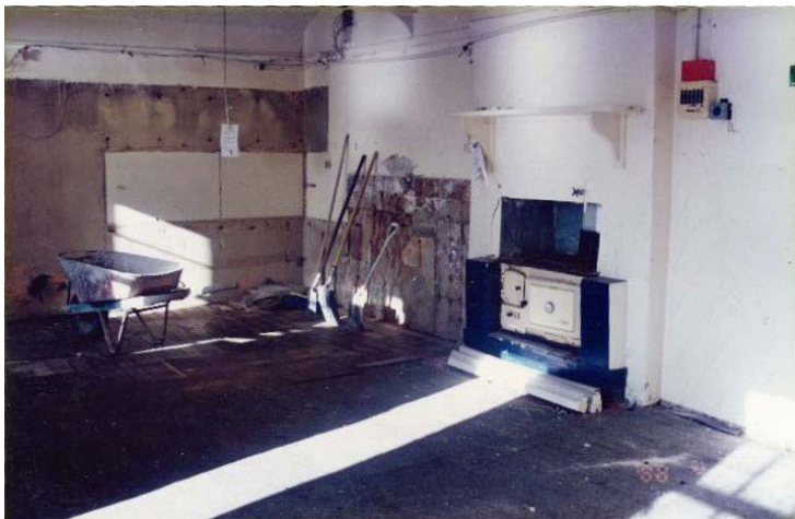
Figure 39 Room B4 looking east, after removal of kitchen sink and cupboards (NPWS 1997)
