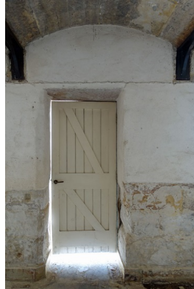
(b) External door to Room B4 (2018)
