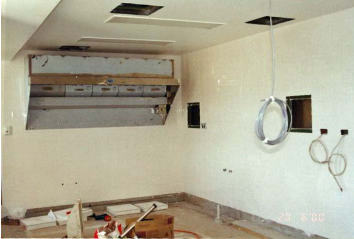
Figure 41 Room B4 looking east, showing over-sheeted walls and ceiling with access hatches (NPWS 2000)
