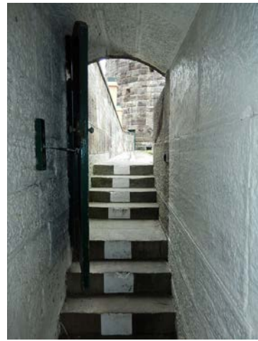
(c) Room B8: door to battery looking north-east
