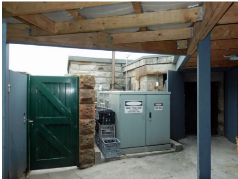
(c) Substation in former slip yard (2016)
