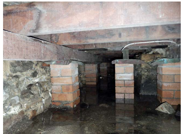
(f) Subfloor area under Room B6/B7 showing standing water at high tide (2016)
