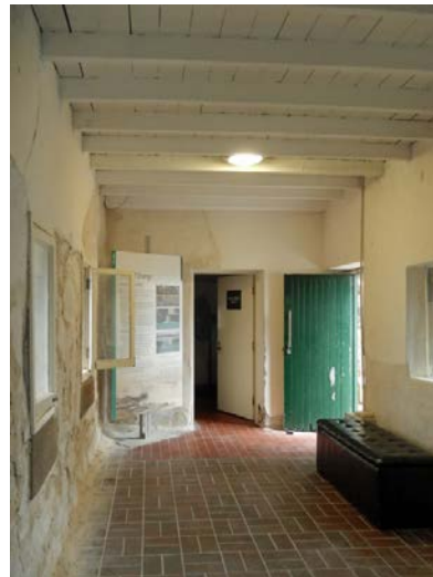
(f) Tide Gauge Room looking south-east to doors to terrace and Room B1
