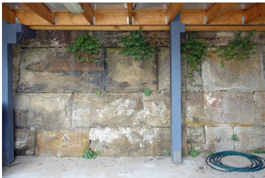
(e) Slip yard shelter and battery wall (2018)
