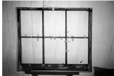
(b) Window sash patched
