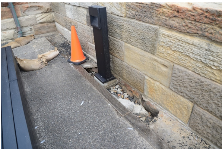
Figure 69 View looking west along the north-west seawall (the terrace), showing damage caused by wave erosion. Note also the recently installed bollard light (Casey & Lowe 2018)
