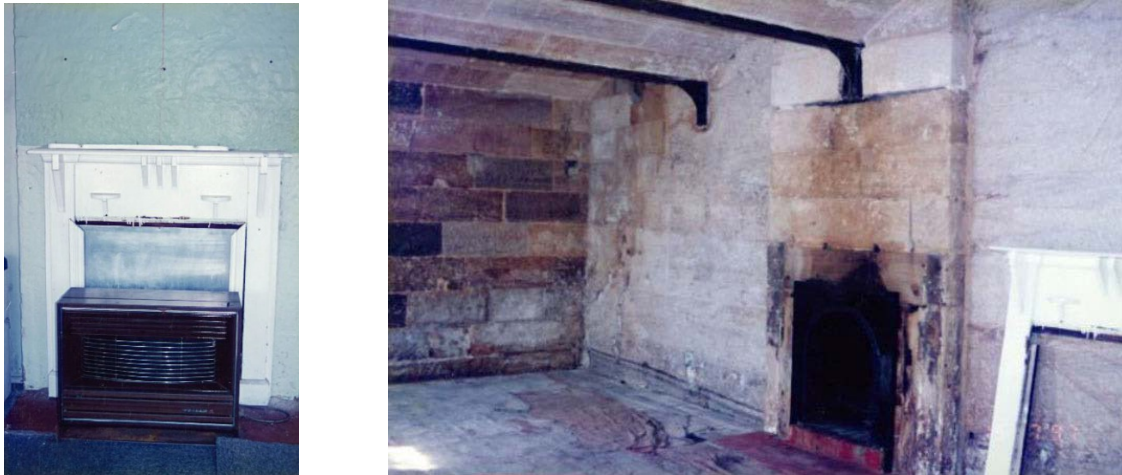
Figure 43 Room B5 fireplace detail (left), and Room B5 looking east (right), after render removal. Note the timber chimneypiece removed from the fireplace (NPWS 1997)
