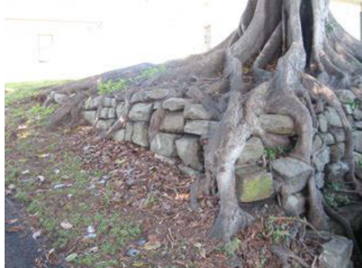
Figure 9: Port Jackson Fig roots Port Jackson fig roots morphing with an historic sandstone retaining wall near the barracks building on the southwestern tip of Goat Island. (Dan Tuck 2007)
