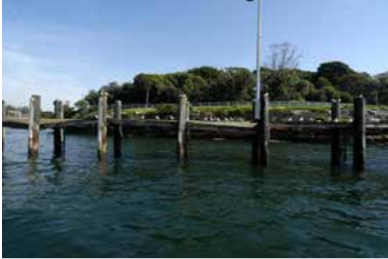
Detail, Wharf Mooring floating plant, showing collapsing decking
