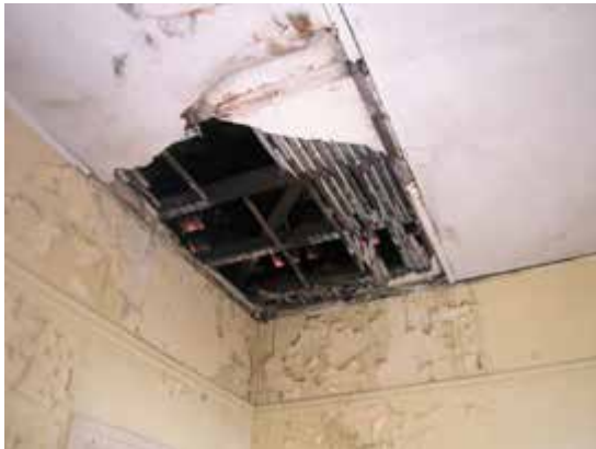
Damage to plaster ceiling of living room, showing exposed timber battens, Residential Cottage No. 3
