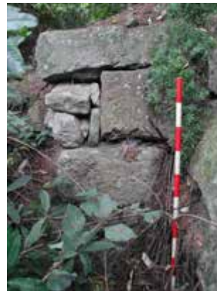
Presumed Blacksmith's Shop site (67). Section of the masonry wall abutting the bedrock outcrop that the cuts have been made into. View to the north.
