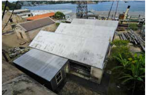
Detail of roof and east extension of Colonial Magazine from above, to east
