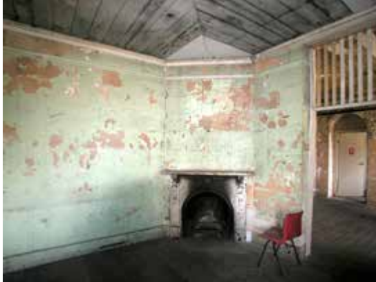
Interior, Water Police Station. Note early 20th century alterations: mantelpiece and screen, wider doorway opening
