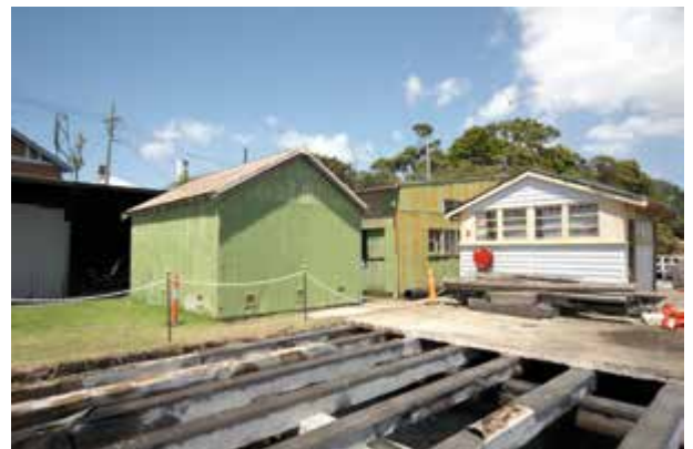
North elevation of Firefighting building behind MSB B456 (57) and corrugated iron shed (56)
