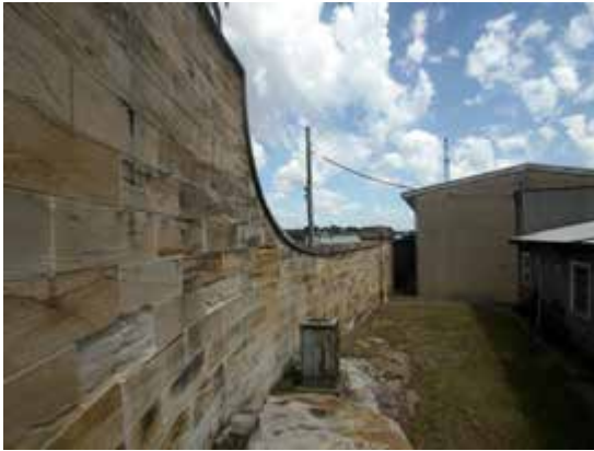
Fortified wall and entry from northern side looking west past item 1a towards entry
