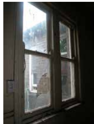
Living room windows, Residential Cottage No. 3. Note broken glass.
