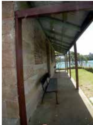
Water Police Station, view along verandah to east elevation. Bricked-up window visible in foreground.
