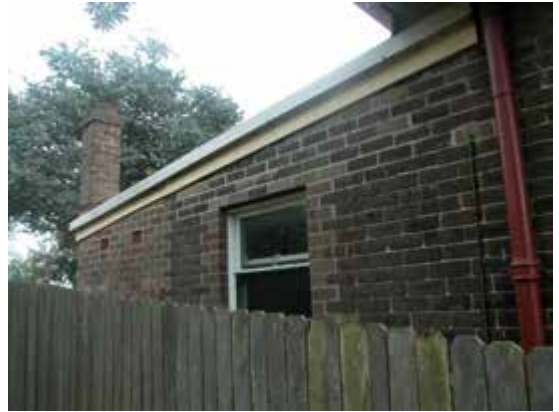
Detail, rear (west end) of south elevation, showing alterations to brickwork indicating insertion of new window, and brick rear laundry extension with chimney
