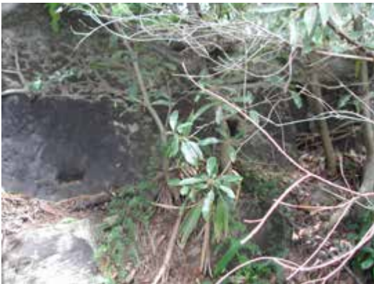
Presumed Blacksmith's Shop site (67). View of the masonry wall to the north of bedrock outcrop. The wall is in poor condition and hidden behind thick vegetation. View to the north.
