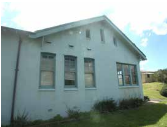
Fire Brigade Barracks, detail of east elevation. Set of three windows at right are clearly a later addition.
