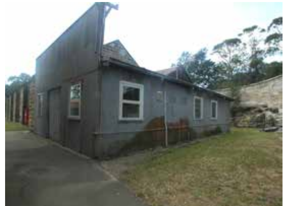
West and south elevations of the Southern addition to the Queen's Magazine looking north from the entry in the Fortified wall (71)
