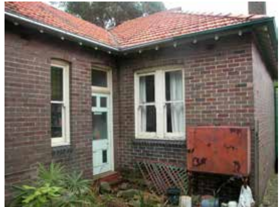
View of rear of southern elevation and door opening south from rear hall
