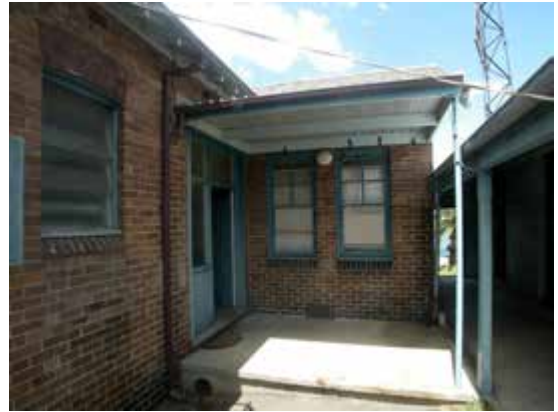
Fire Brigade Barracks, detail, south elevation, area around entry door. Cottage 46a verandah to right.
