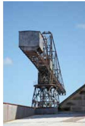
Close view of top section of Hammerhead crane including crane driver's cabin
