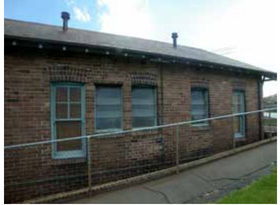
Fire Brigade Barracks, detail of western end of north elevation, showing window alterations
