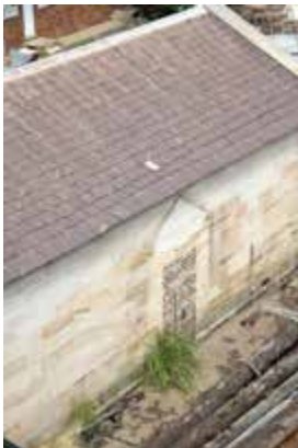
Cooperage north elevation showing bricked up entry door which once connected to a covered way leading to the Colonial Magazine.
