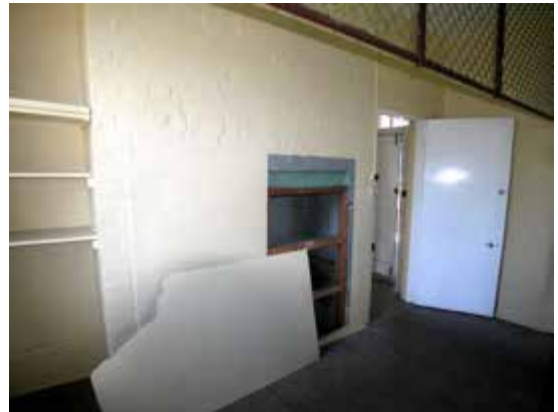
Southern room of cottage, showing later door, original hearth with later shelving, part of clothing racks, part of entry vestibule and main entry door visible through the door
