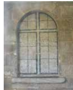
Water Police Station, detail of painting to blind window on south elevation (within the weatherboard addition).
