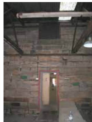
Door into southern elevation of Queen's Magazine, interior of Southern addition to Queen's Magazine
