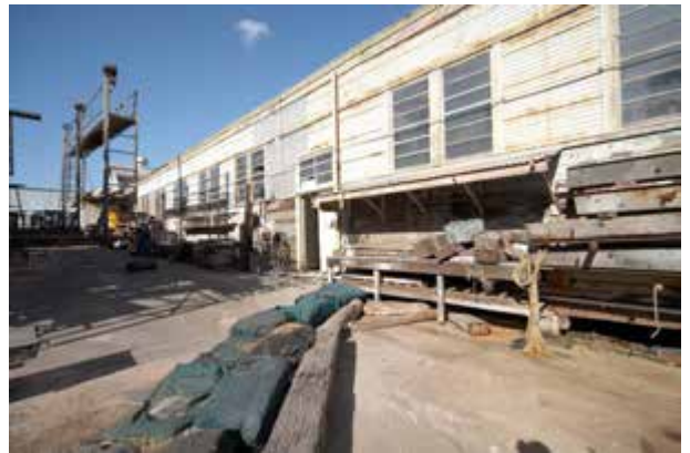
Repair workshop, east elevation at left (slipway workshop building in foreground at right)
