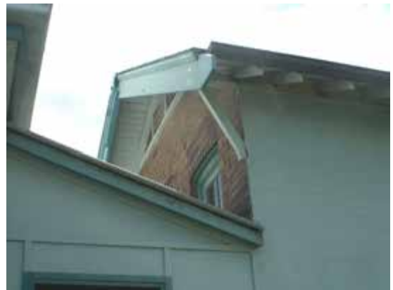
Detail, Fire Brigade Barracks, junction of verandah roof of Cottage 46a on left with gable end to Fire Brigade Barracks at right
