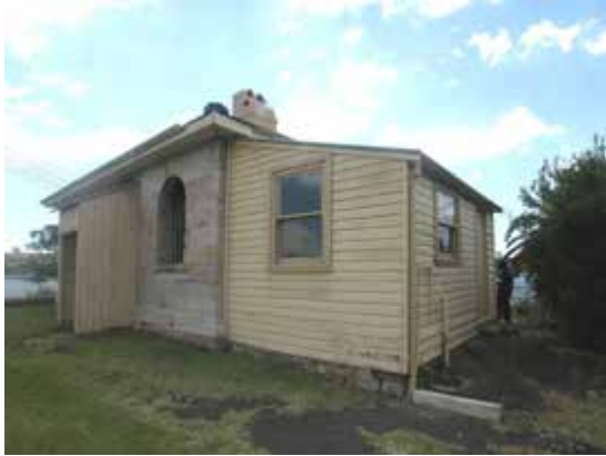
Water Police Station west elevation to right, part south elevation to left, with later weatherboard addition.
