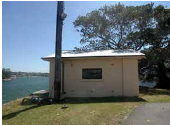
Transformer House (24) with Port Jackson Fig (behind) to southeast of stone jetties (64,65)
