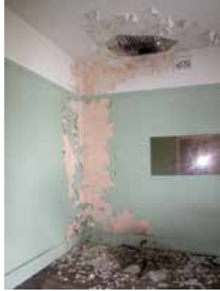
Bedroom with damaged plaster, Residential Cottage No. 3
