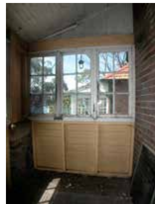
Detail, weatherboarding and timber framed windows to south end of front verandah
