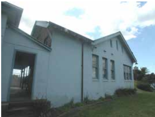
Detail, east elevation, Fire Brigade Barracks, with verandah of Cottage 46a at left
