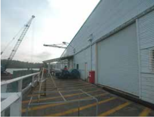
Addition to Ship Repair Workshop in right foreground. The addition is located at the northern end of the Ship Repair Workshop.
