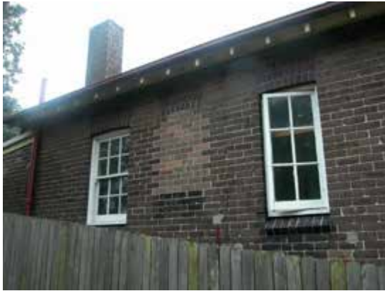
Detail, south elevation, Residential Cottage No. 4, showing brick infill of former window opening
