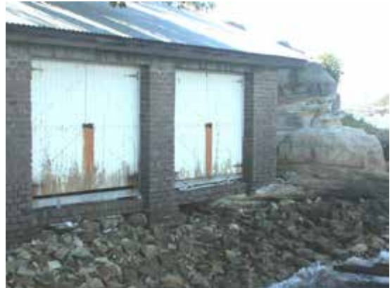
Detail, 3-door boatshed, showing erosion of brickwork.
