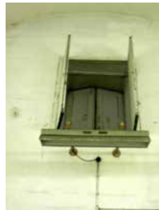
Double timber shutters to north end of Queen's Magazine, taken from interior
