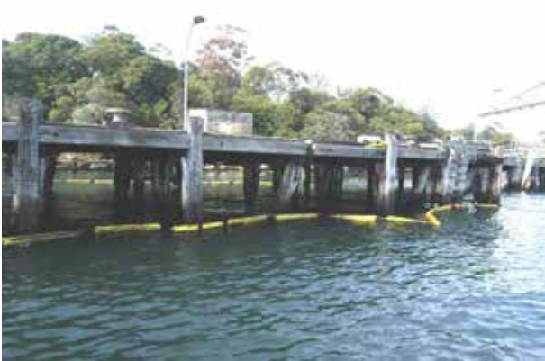
Coal bunker platform at northern end of Broadside wharf, from the west
