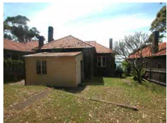
Rear elevation and south elevation from west, Residential Cottage No. 2, showing later rear weatherboard addition
