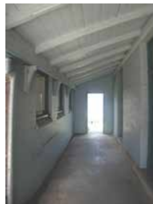
Verandah of Cottage 46a and part of south elevation of Fire Brigade Barracks 46b on left
