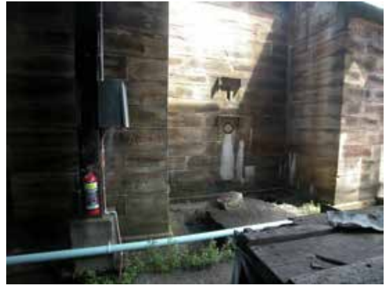
Detail, west side of Scow shed interior, showing floor of Scow shed excavated away from the east wall of the Queen's Magazine
