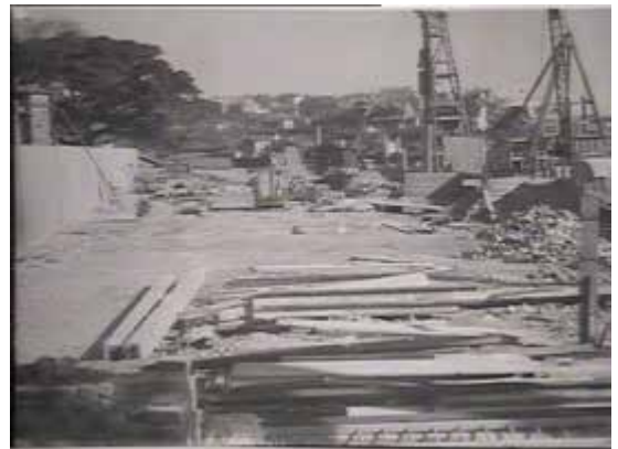
1946 photo of construction of the Ship Repair Workshop (State Library Image No. GPO 1 - 10116)
