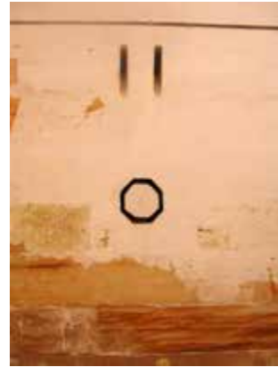
Baffled vent from interior of Queen's Magazine. Note damage from damp penetration below.
