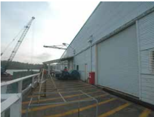
Central and southern section of Broadside wharf, adjacent to Ship Repair Workshop (1)
