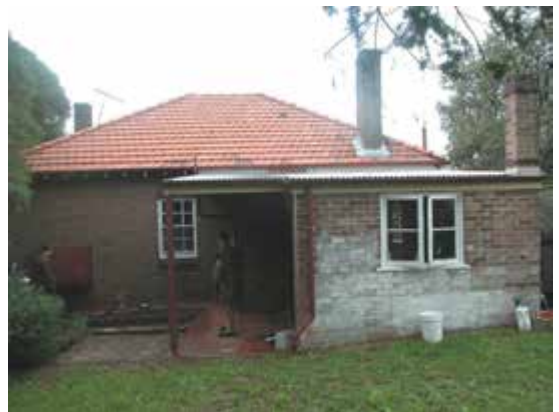
Rear (west) elevation, Residential Cottage No. 4, showing 3 chimneys to roof, and brick rear laundry extension
