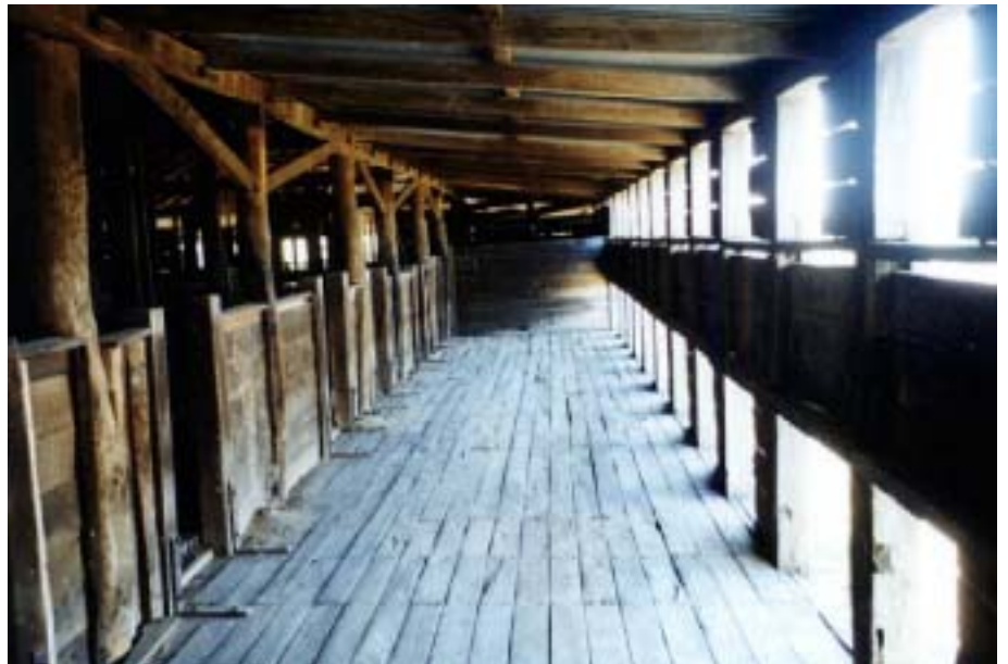
Figure 45 The blade board [south side]. Rebates and bolt holes on the upper face of the posts accommodated the beam that supported the first phases of overhead gear. It is likely that hessian bags would have hung over the windows. PG 2001 photograph
