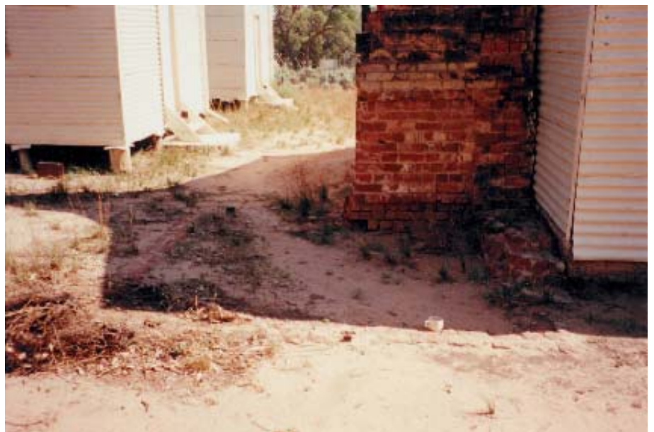
Figure 95 Brick foundations can be seen adjacent to the existing chimney in the Cookhouse building. This was the former bread oven site. SMT 2001 photograph
