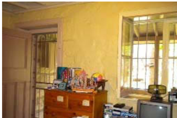
View of room G2 looking towards the front door and the verandah beyond. Source: Author October 2010.
