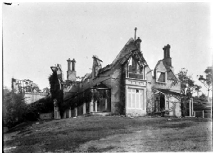
Greycliffe from the north east gutted after the 1897 fire with just the stone walls standing. Source State Library NSW Ref perier_34367r
