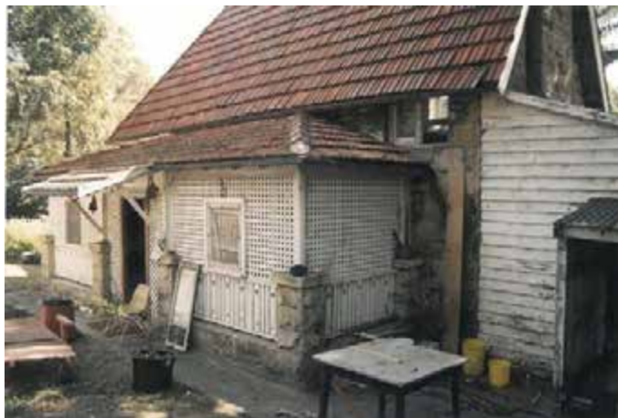
View of the rear of the cottage in 1992 showing the condition of the extension originally constructed by the Park Trust and later altered and filled in. Source: Schwager Brooks and Partners 1992.
