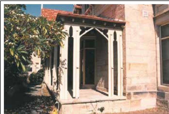
North east verandah with enclosure removed by NPWS.
