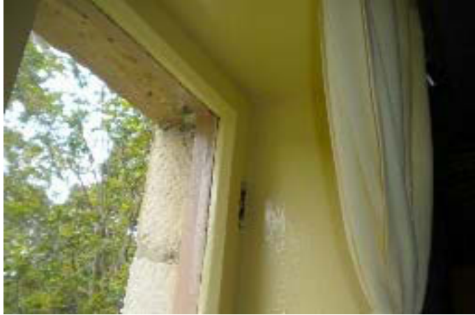
Detailed view of the front window in G1 showing the simple rustic casement and frame in the deep reveal. Source: Author October 2010.
