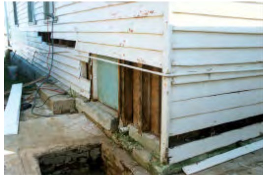
Fig MH26.10 The works uncovered a door to the laundry covered over by boards. NPWS MAINTENANCE FILE F/590 - 2001
