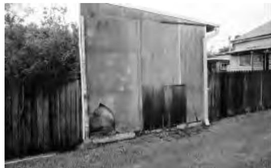
Fig MH31.24 The end wall of the shed is in a substantially poorer condition. PAUL DAVIES PTY LTD 2002
