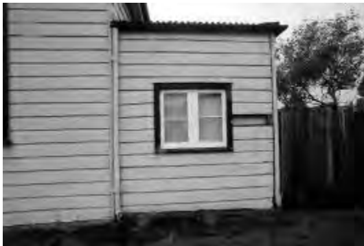
Fig MH31.10 Detail of verandah enclosure from south east. PAUL DAVIES PTY LTD 2002
