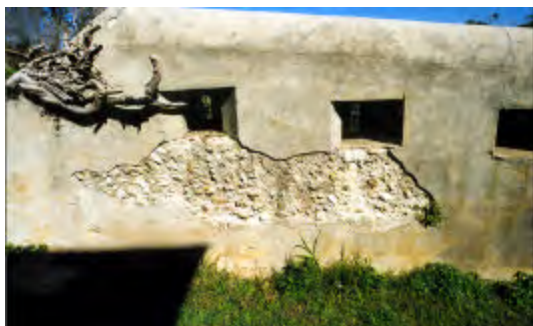
Fig 4.11 The defensive wall associated with the area of the moat around MH29 showing the “loop holes”. The mass concrete walls are in a relatively poor condition and are in need of conservation. Such things as plant growth, damp and being covered by soil are causing these important elements to deteriorate. PAUL DAVIES PTY LTD 2002
