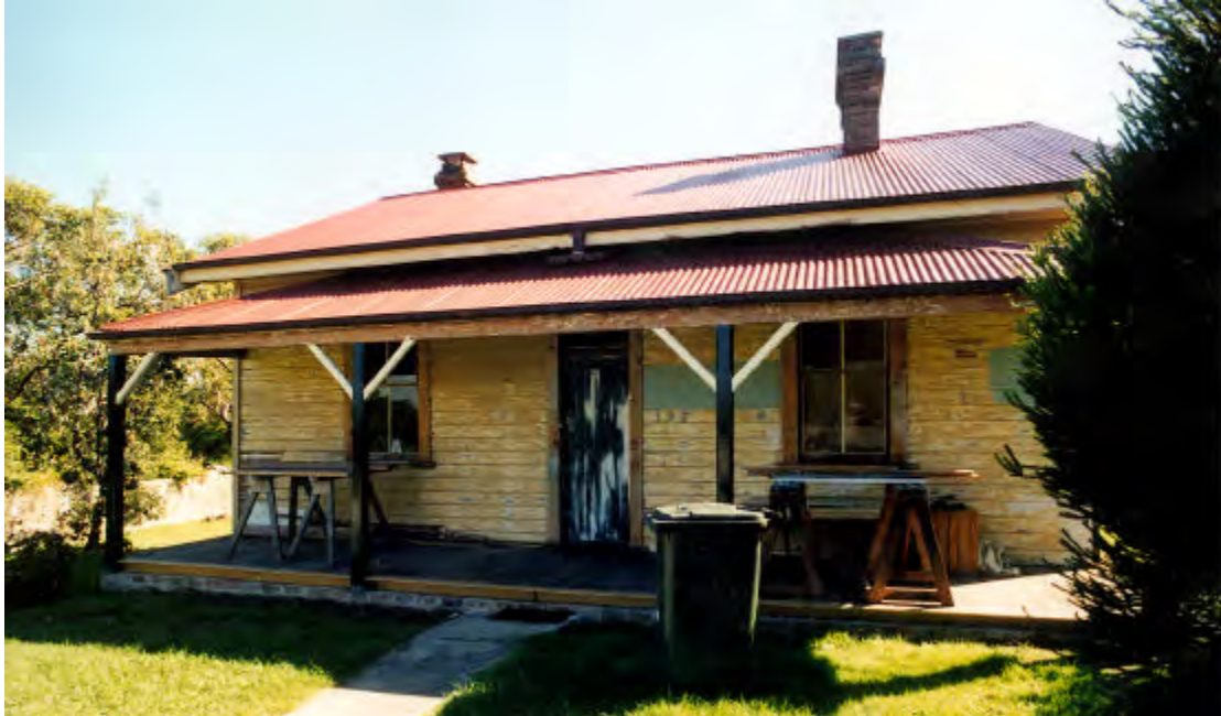
Fig MH30.2 The front (south east) elevation showing verandah and front wall in process of repair works. PAUL DAVIES PTY LTD 2002
