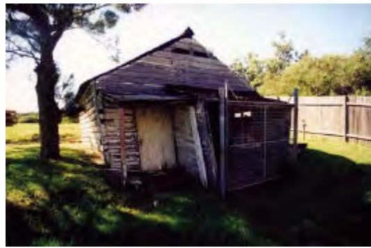
Fig MH34.4 Photo of front of coal store showing general structural and cladding failure. PAUL DAVIES PTY LTD 2002
