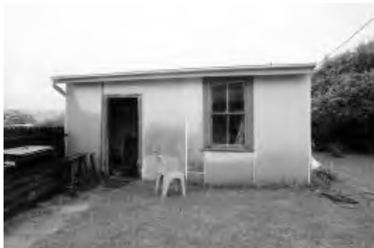
Fig MH31.23 The rear shed with a salvaged (or original) four paned window and ledged door. The FC sheet appears in fair to poor condition. PAUL DAVIES PTY LTD 2002
