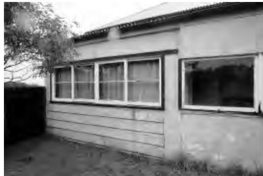
Fig MH31.11 Detail of verandah enclosure showing sliding windows and FC sheet adjacent. PAUL DAVIES PTY LTD 2002
