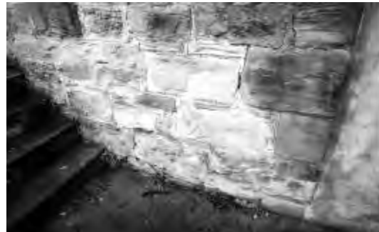
Fig MH29.17 Stone wall requiring some level of repointing. PAUL DAVIES PTY LTD 2002
