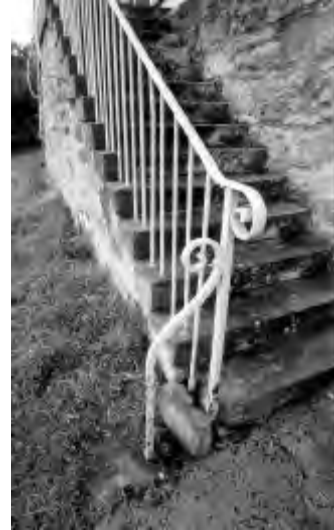
Fig MH29.20 External stairs showing corrosion damage to wrought iron and subsequent cracking to stone treads. PAUL DAVIES PTY LTD 2002
