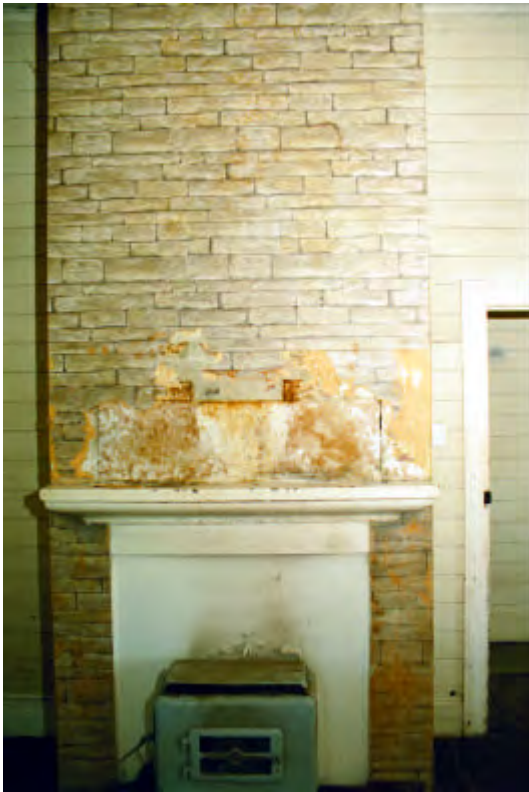
Fig MH26.9 The fireplace and chimney in 26.03 showing that the original finishes had been stripped to bare stone substrate. NPWS MAINTENANCE FILE F/590 - 2001
