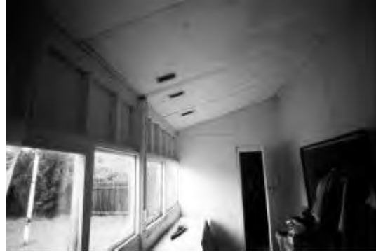
Fig MH31.15 Interior of verandah enclosure showing that original exterior cladding removed in favour of FC sheet. Note the low window heads. PAUL DAVIES PTY LTD 2002
