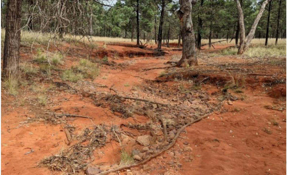
Figure 17 Looking downstream (west) to where the proposed conservation fence line intersects with unnamed creek #2 – significant erosion/deposition within the creek can be seen
