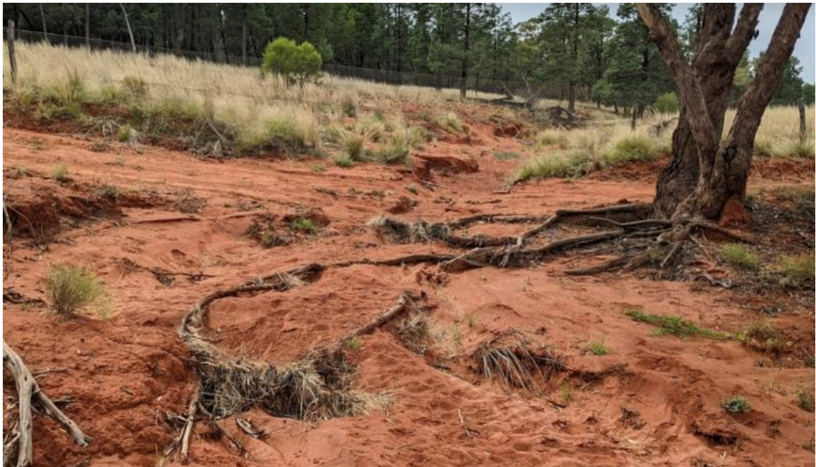
Figure 16 Looking upstream (east) to where the proposed conservation fence line intersects with unnamed creek #2 – significant erosion/deposition across the road and within the creek can be seen
