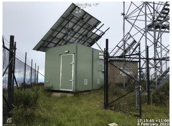
View to the existing equipment shelter facing north-east
