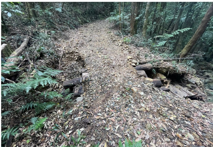
Figure 45 Damaged log gully crossing requiring replacement
