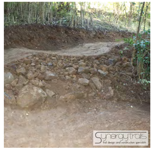
Rolling Dip with Hardened Spill Way
