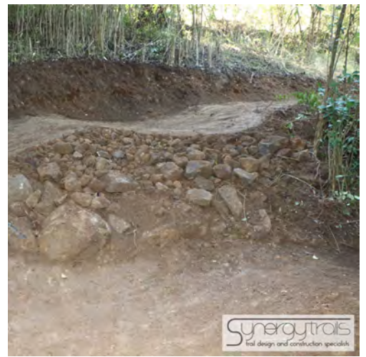
Rolling Dip with Hardened Spill Way
