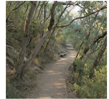
Aged exposed aggregate concrete path
