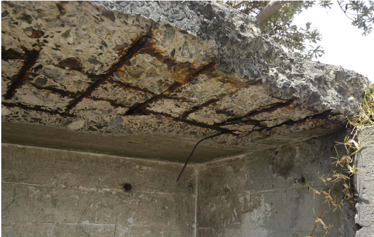
Figure xi An example of severe concrete deterioration at South Head which will in time if not treated cause structural failure of the element.
