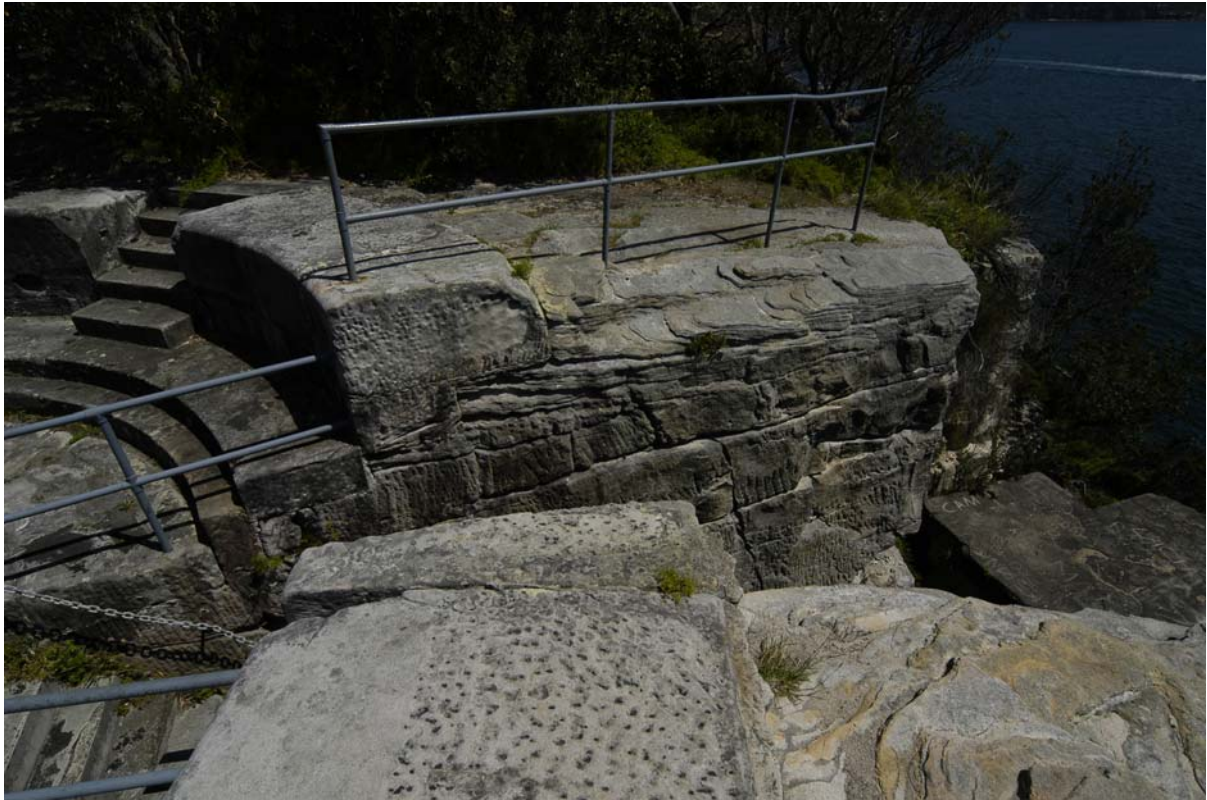
Figure xix Outer Middle Head showing a location where secure fencing is required as it is easily accessible and the drop-off is unexpected and dangerous. While the fencing is not complete in that it does not return, it marks a dangerous location adequately to warn visitors not to proceed past the edge of the fence. This is an excellent example of when to provide barriers. In contrast, the chain to the left of the picture is a handrail down a steep set of steps and it is not a suitable element and should be removed as it presents a danger to users in itself.
