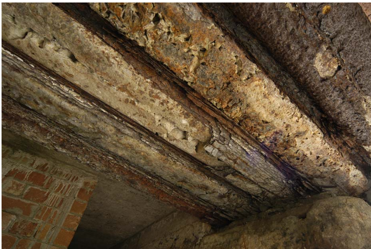
Figure xii An example of severe steel corrosion to Barlow Rail roof supports at South Head.
