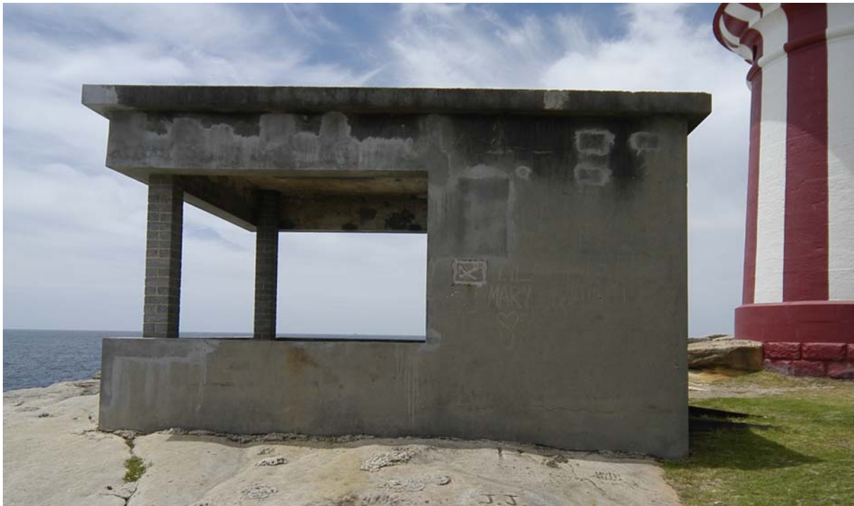
Figure xii Another example from South Head where extensive reconstruction of concrete has taken place and failed steel posts have been replaced with more robust concrete blocks to conserve this prominent concrete element.
