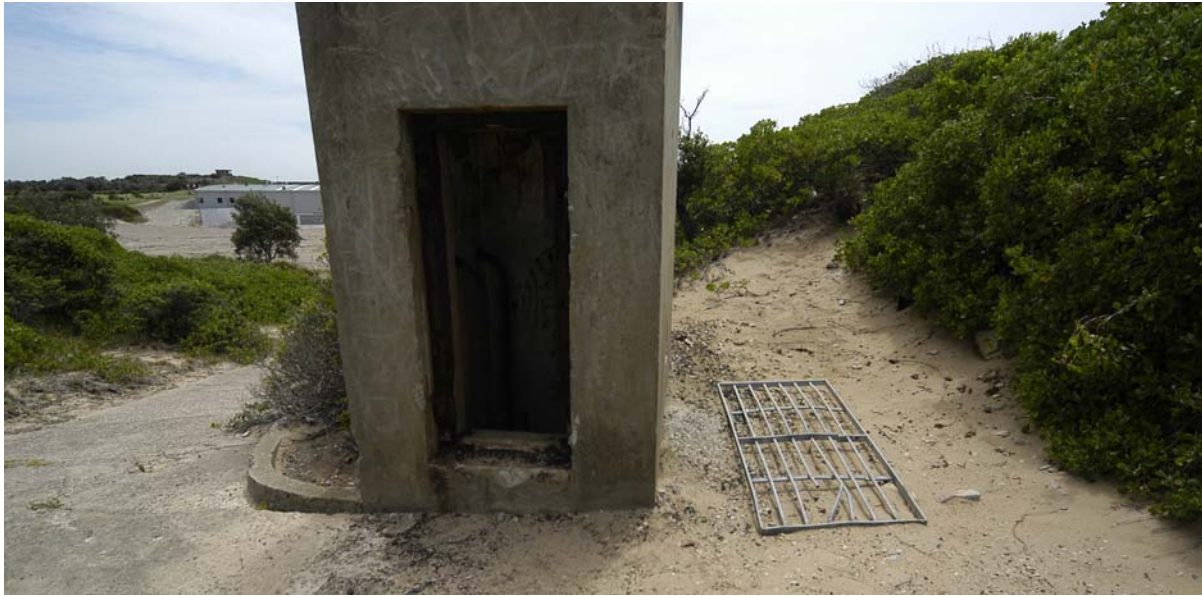
Figure xv A severe example of vandalism to gain entry to the below ground areas at Cape Banks. This not only requires repair but presents a serious risk to other visitors as there is a substantial drop with the gate removed. This type of activity needs to be monitored regularly and responded to quickly.
