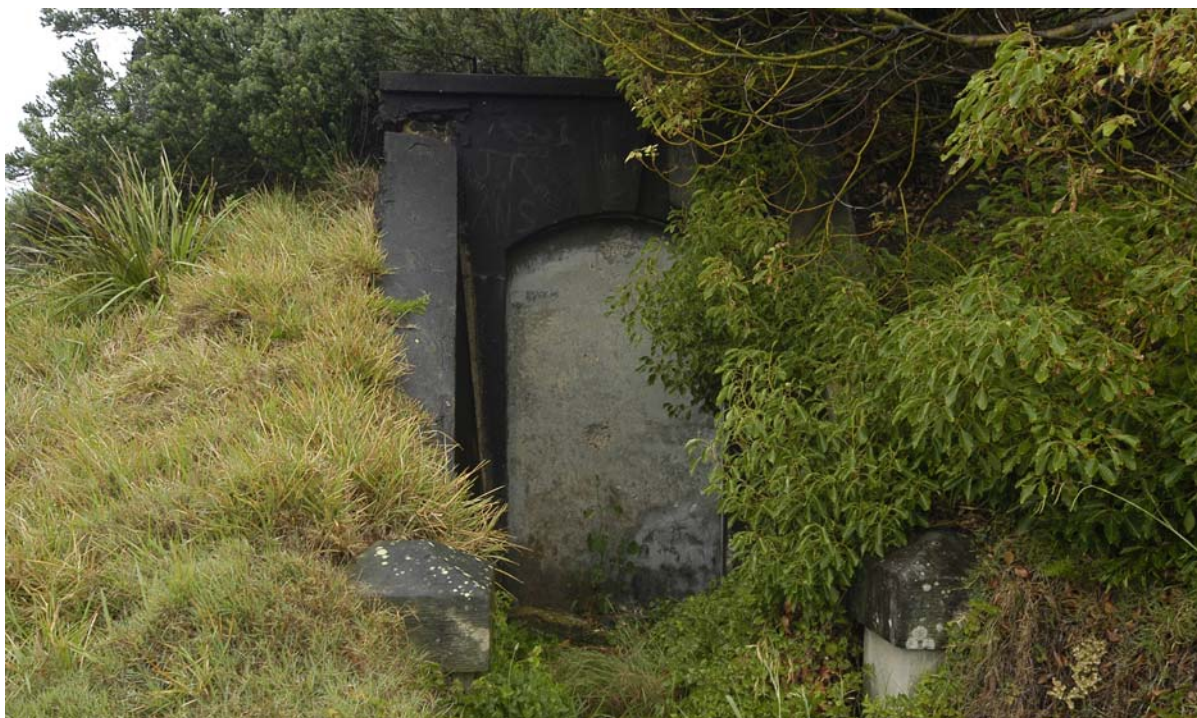
Figure xvii Entry to Green Point tunnels (blocked) with extensive undergrowth that requires maintenance.
