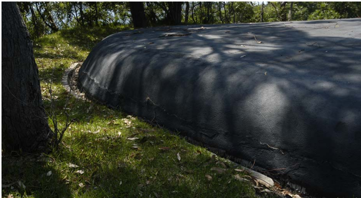
Figure xvi Membrane applied to roof of armoured casemate as part of previous maintenance works. Note the edge cracking and failure of the membrane through movement. Ongoing maintenance of areas such as this are essential to ensure that the fabric is conserved and that best value is obtained from conservation works.
