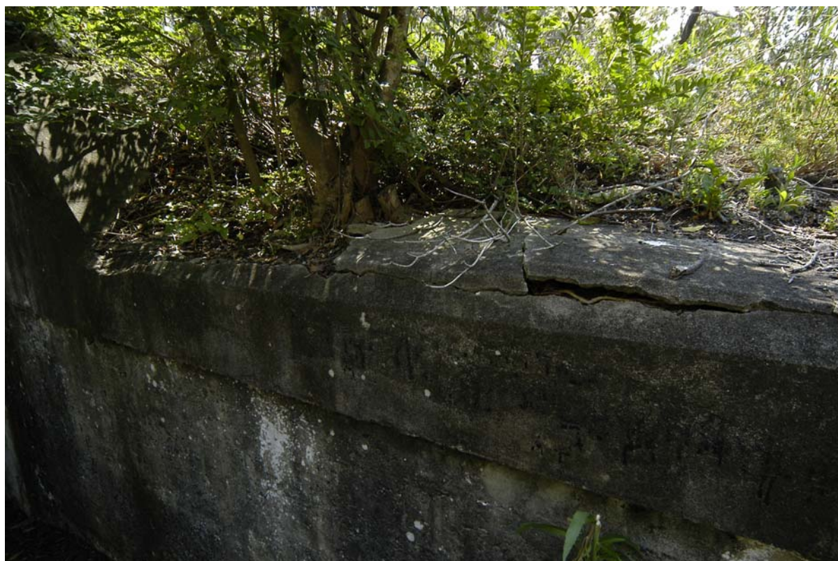
Figure xiii Example of damage from self-sown and unwanted plant growth around edges of structures. Inner Middle Head fortifications.
