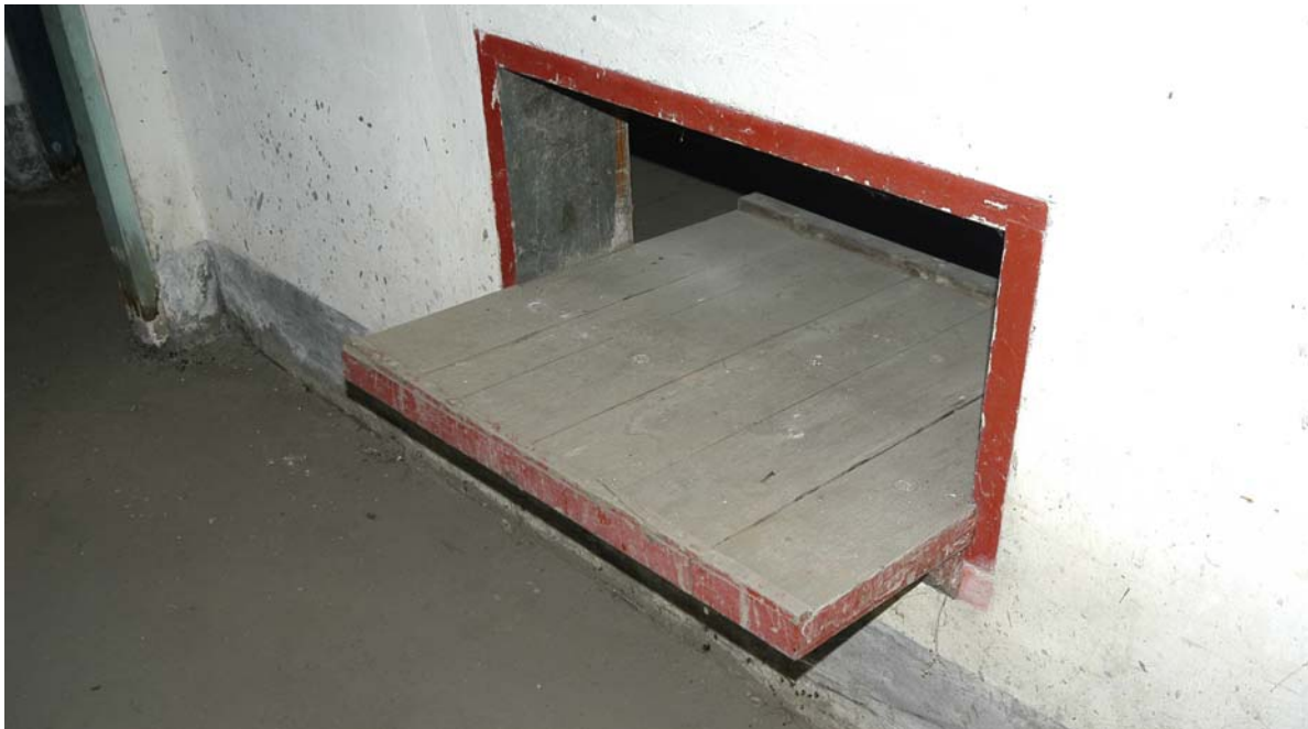
Figure x Conservation work to timber elements in the underground magazine at South Head to reinstate deteriorated elements based on careful research and site investigation.
