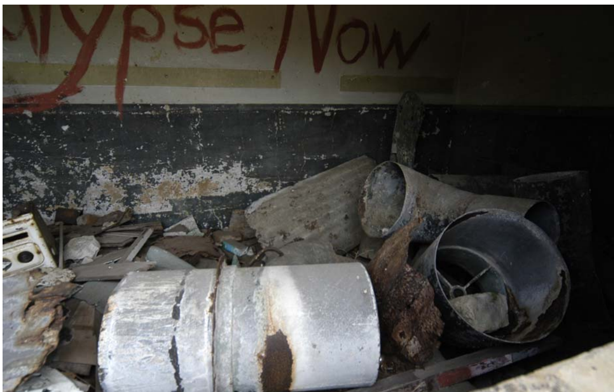
Figure xiv Cape Banks structure interior that is easily accessible and full of rubbish from the site, note the graffiti that features as this site.
