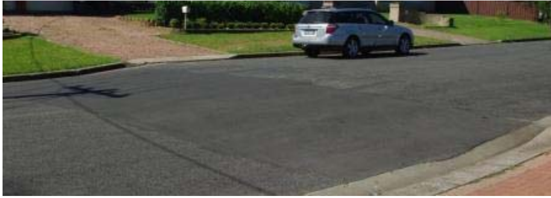
Figure 8-6. Result of mine subsidence in Tahmoor. The vertical offset is >500 mm on either side of the patch in the road.
