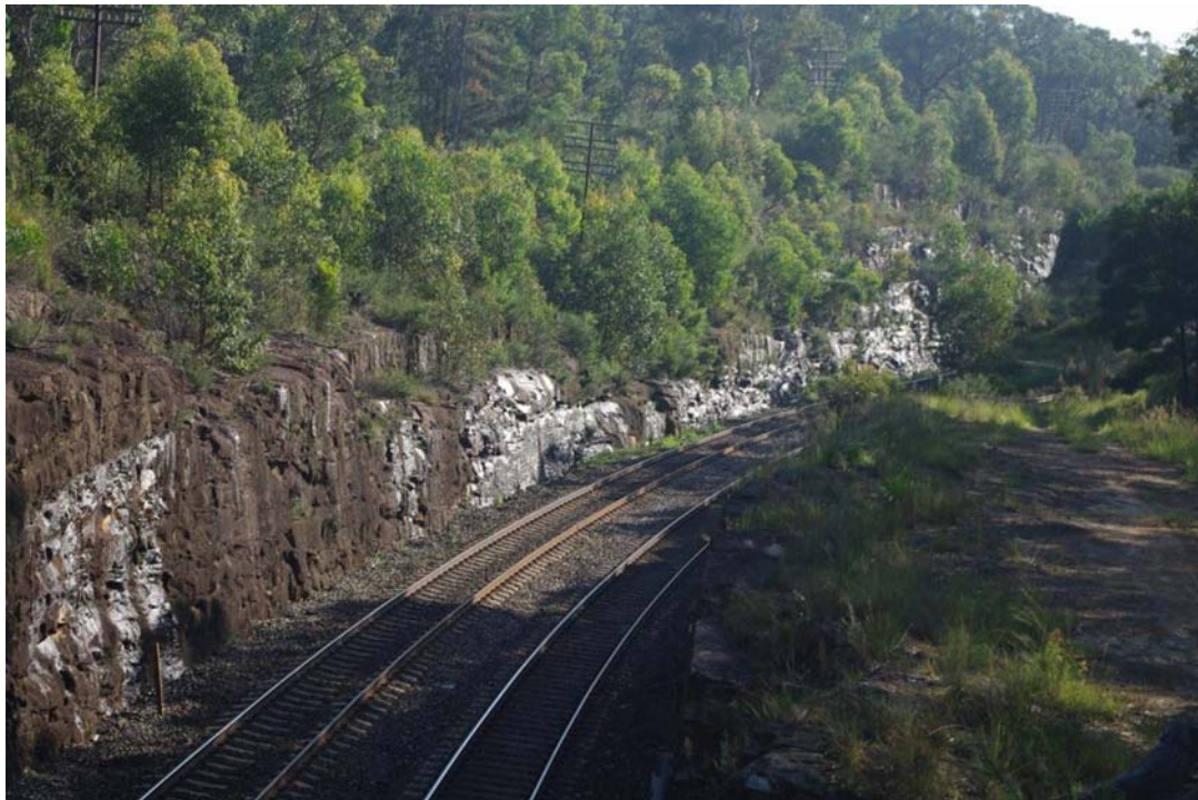
Figure 6-3. Groundwater emerging from the east-facing slope on the railway cutting at Bargo River Rd.
