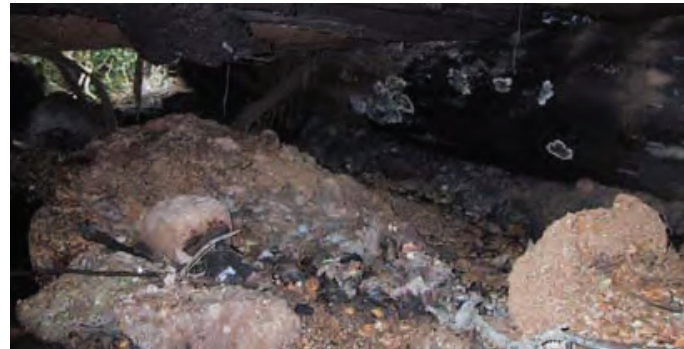
Figure 22. Spoil in the drainage feature beneath a bridge
