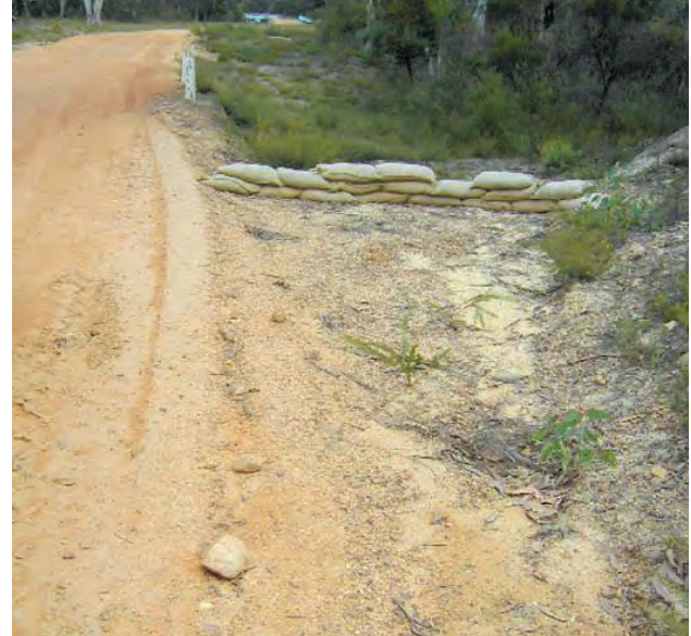
Figure 37. A sandbag sediment trap with a spillway in the outlet of a table drain
