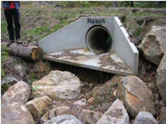
Figure 26. Scouring beneath a headwall
