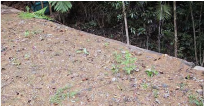
Figure 21. Soil entering a drainage feature from the pavement of a bridge surface
