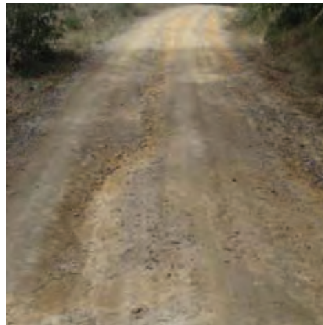
Figures 1 and 2. Rilling and scouring of the road surface indicating poor drainage
