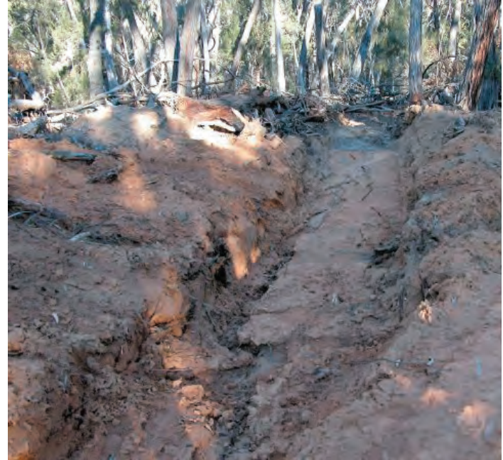
Figure 3. A mitre drain requiring repair and reshaping
