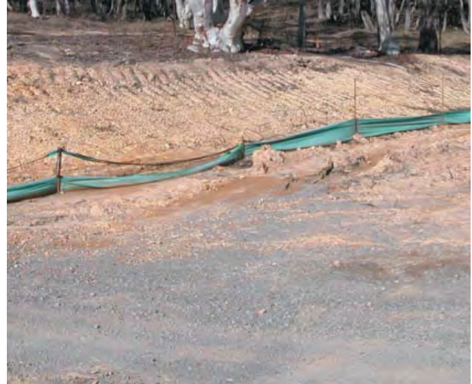
Figure 35. A poorly maintained sediment fence
