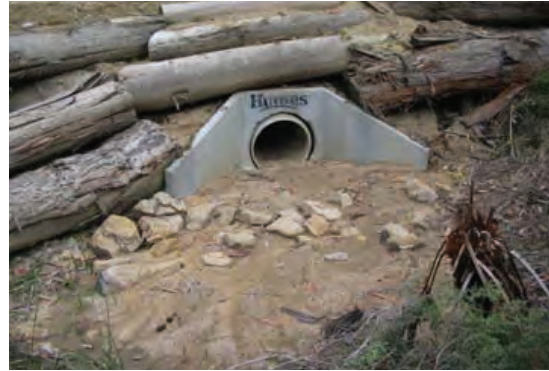
Figure 25. Culvert outlet requiring clean-out and stabilisation – head-wall placement too low resulting in erosion from the pavement
