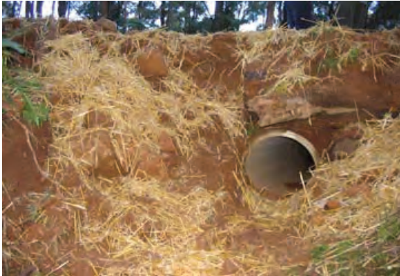
Figure 24. Poor stabilisation of batter
