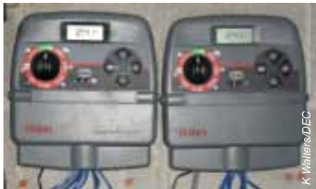
Irrigation controller at Greenway Park stormwater reuse scheme, Cherrybrook
