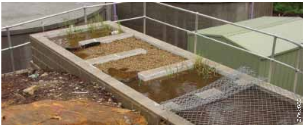
Sand filter and wetland
