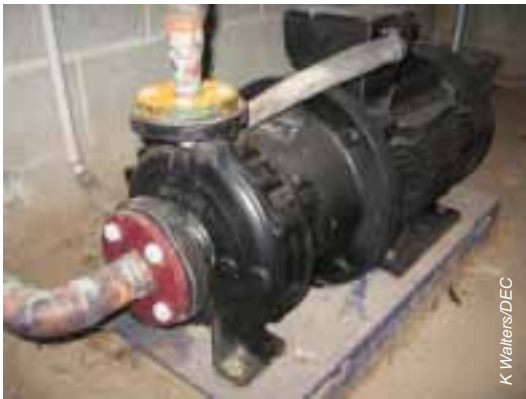
Stormwater pump at Greenway Park stormwater reuse scheme, Cherrybrook
