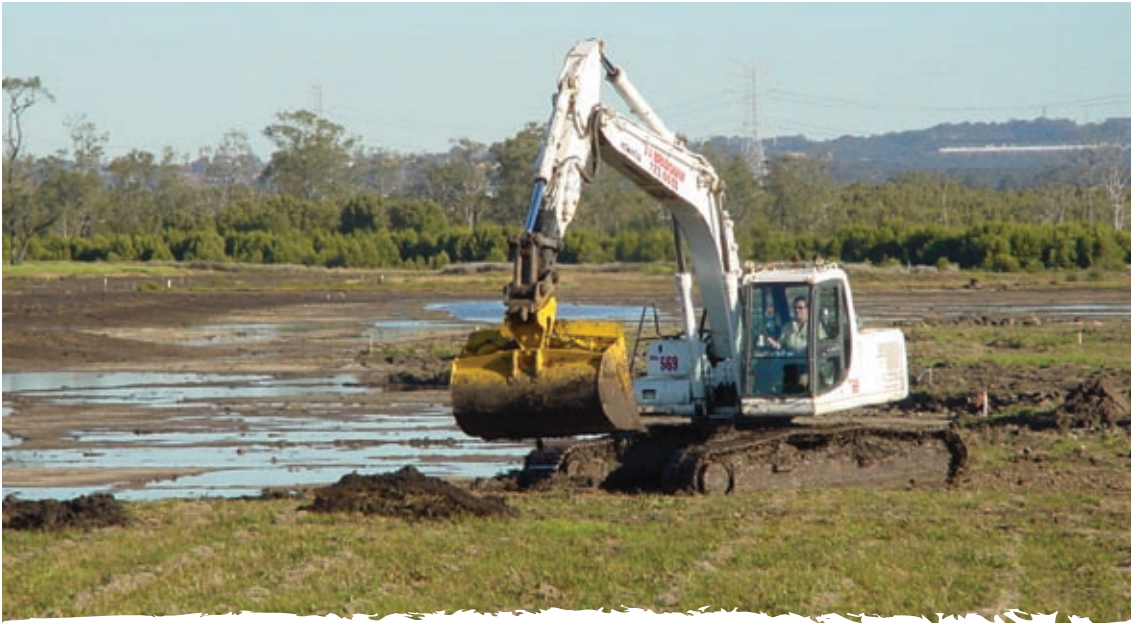
Construction of saltmarsh as part of the Kooragang Wetland Rehabilitation Project (Kooragang Wetland Rehabilitation Project)
