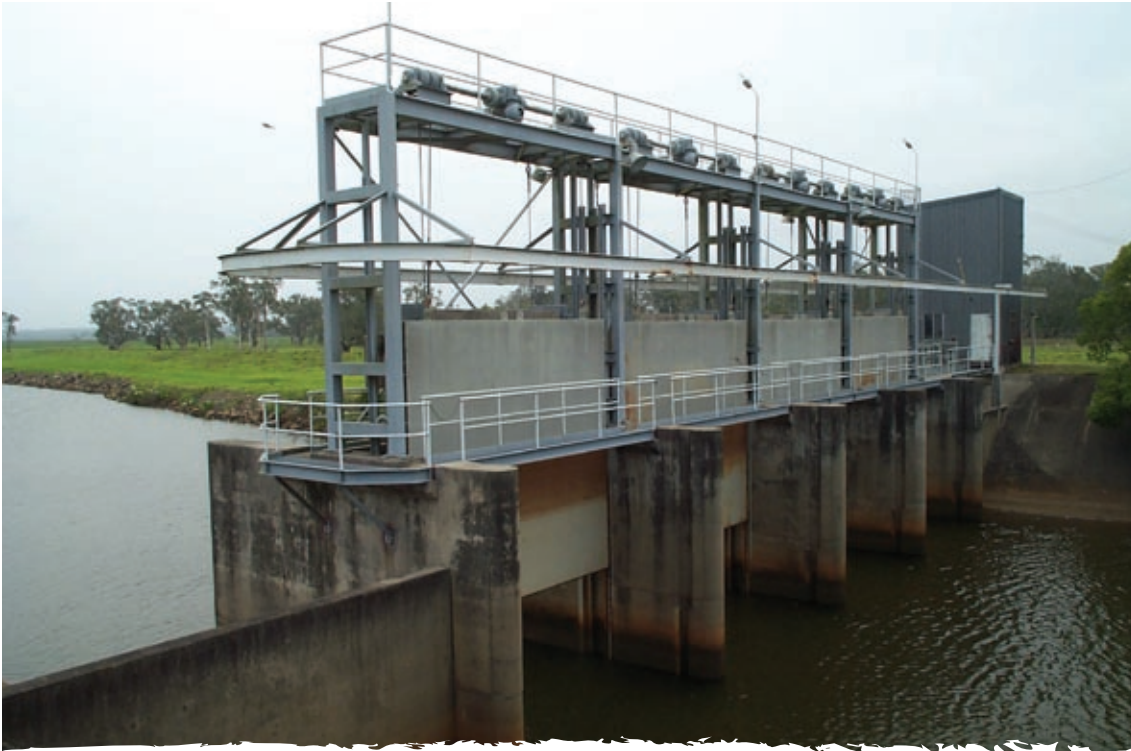
Floodgate at Macleay River (DECC)
