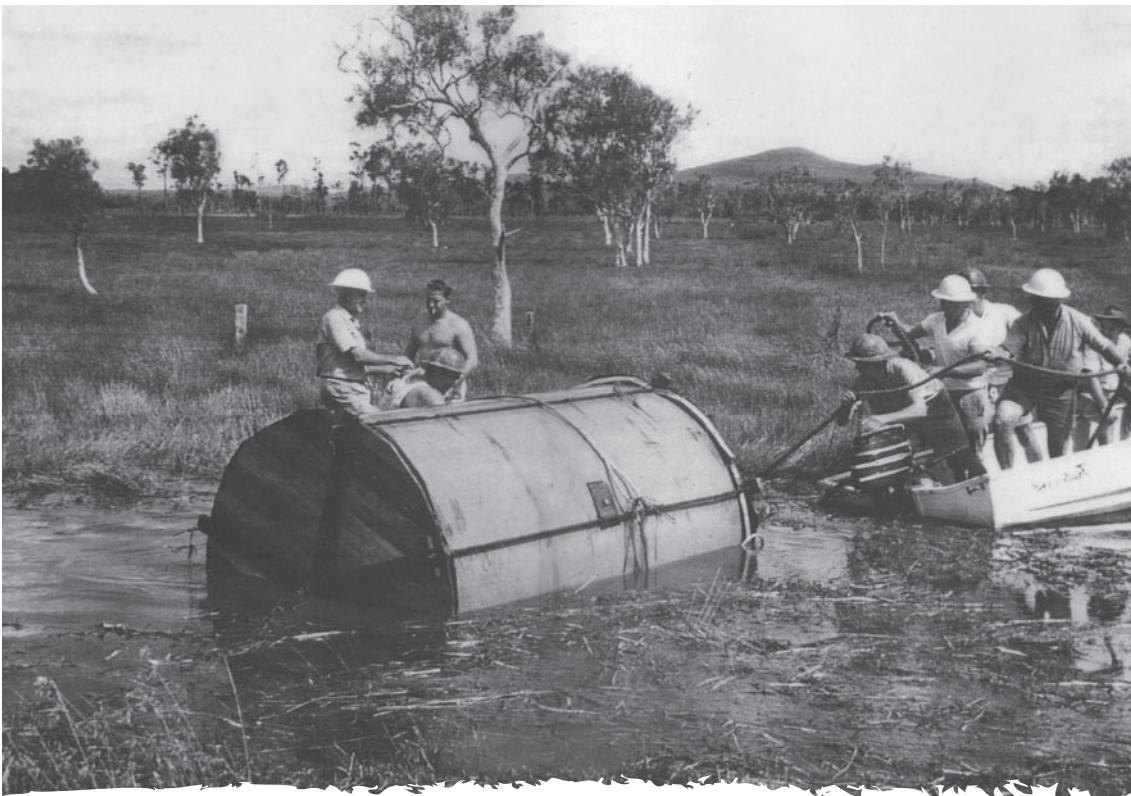
Pipe being floated over a wetland during the 1966 construction of the Taloumbi Radial drains, that now drain into Lake Wooloweyah (Clarence Valley Council)
